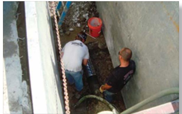
Predictable state funding is critical to address State of Good Repair projects- West Division water main break in 2013.
