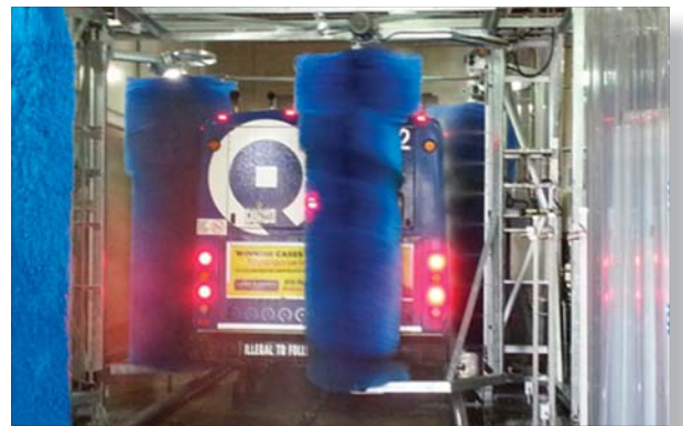
In 2012, Pace replaced the bus wash system at Heritage Division. Portions of this building are nearly 90 years old and dates back to 1926.
