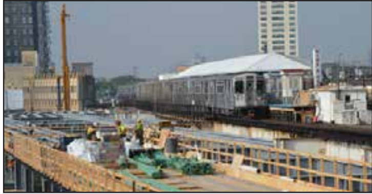
Approximately 2,200 feet of elevated tracks, signals and supporting infrastructure are being relocated as part of the Wilson Rehabilitation.
