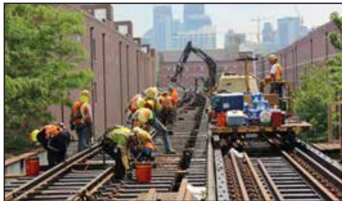
Construction crews replacing track structure as part of the Ravenswood Connector Rehabilitation Project.
