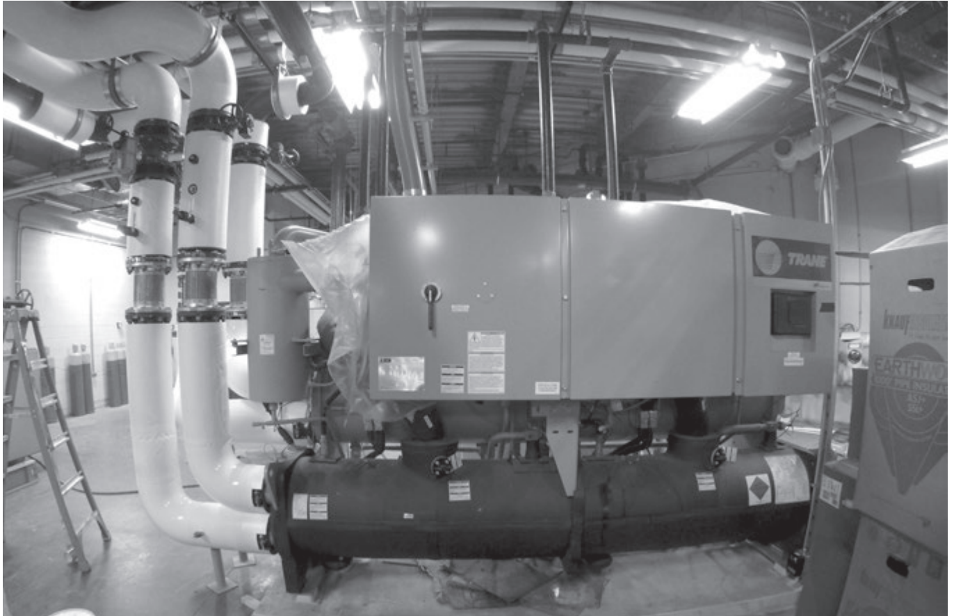
Skokie Courthouse – New Geothermal Chiller
