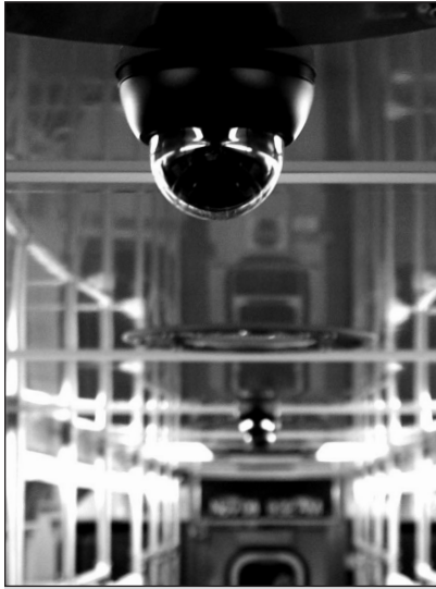
CTA began retrofitting most of its existing rail fleet with surveillance cameras this year. By 2015, more than 8,300+ cameras will be available across the rail fleet making it the most comprehensive rail system camera network among U.S. transit agencies.
