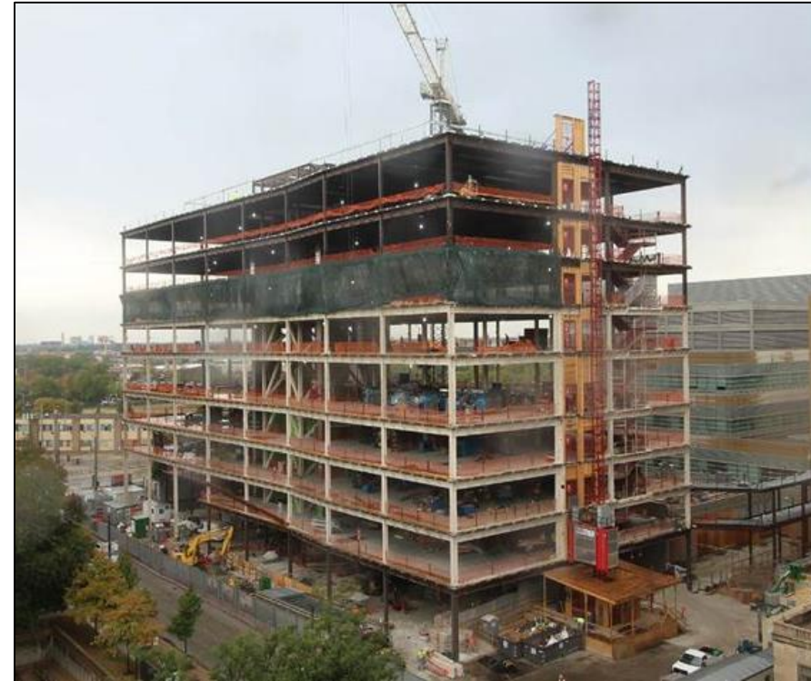
Cook County Health and Hospitals System – Central Campus Health Center (under construction)
